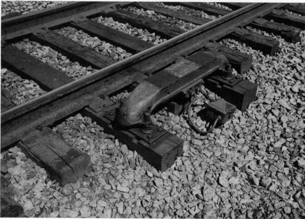
Figure 3. A typical wayside inductor installed in intermittent train stop territory.
